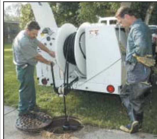
SUCK IT UP: Physical plant plumbers Stephen Klein (left) and Terry Schaefer operate the Shamrock Sewer Jetter that is used to clean sanitation and storm water drains on campus. The high-powered machine has saved time and money compared to formerly paying contractors to do the work.
