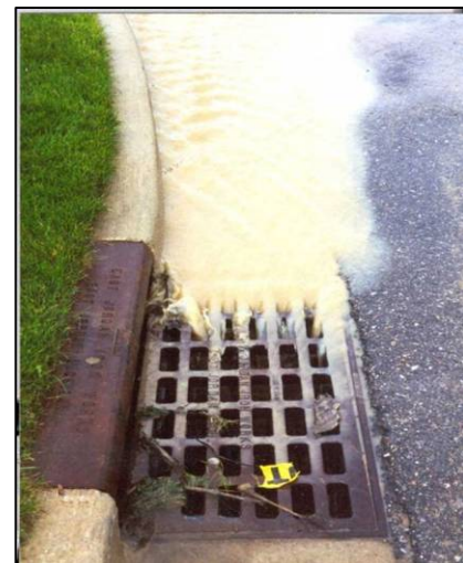
Stormwater carries sediment directly into the nearest waterway. Photo: HRWC files
